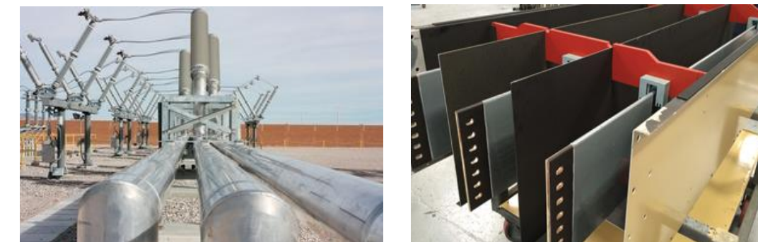
High Voltage Bus
