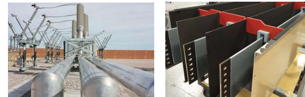
High Voltage Bus
